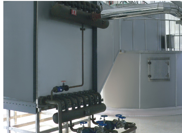
奶粉工程进风加热部分 Air intake heating system for milk powder
